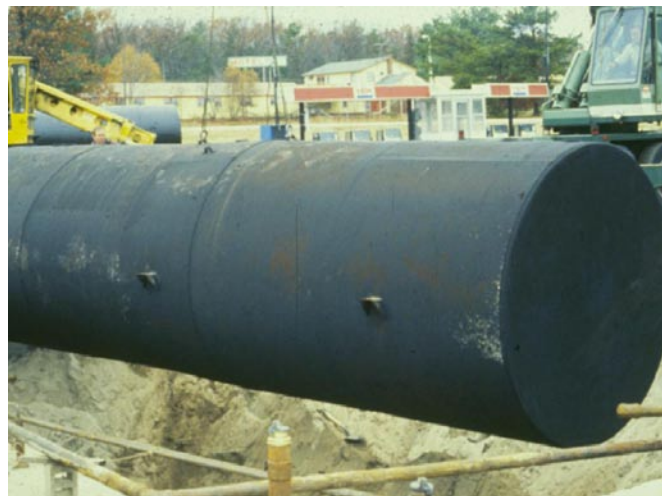
How many of today's UST inspectors can remember seeing a bare-steel UST being installed – legally?
